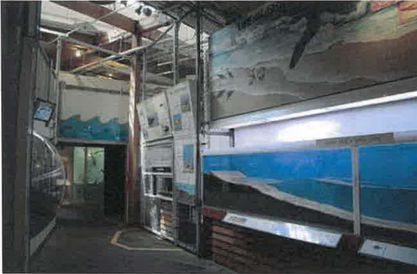
The chain link fencing in the interior of the exhibit has lost its original function of defining space.
