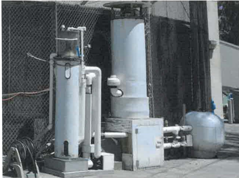
The life support system is in critical need of replacement before the exhibit hall can be remodeled.
